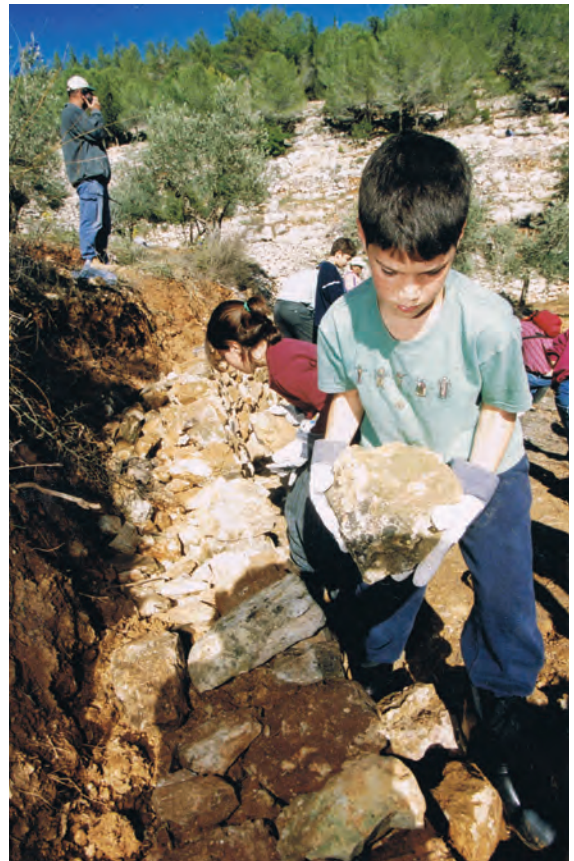
Land designated for a community forest. Terrace restoration in an orchard by the Mevaseret Tsiyon community.
