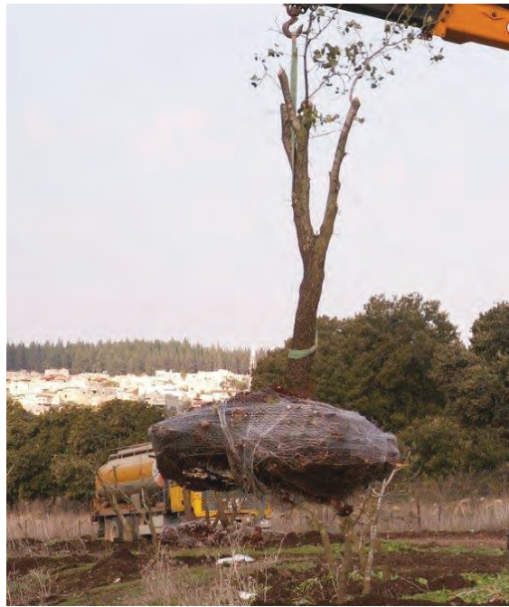
Transplanting mature trees. Using a truck crane to transport and plant a translocated tree in a forest.
